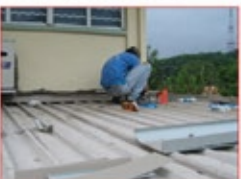
Roof Leak, Water-proofing Works...
